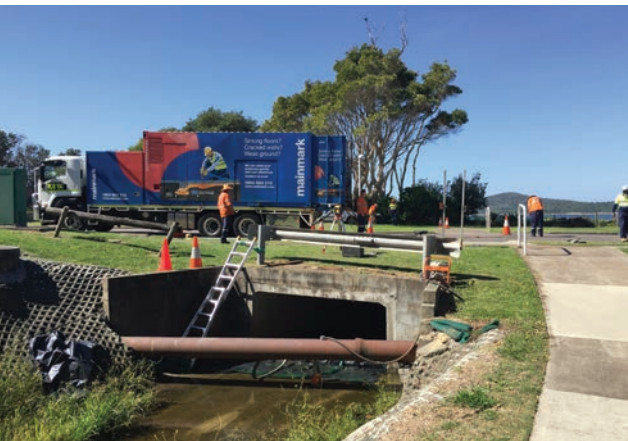
Underground pipeline/culvert raised
